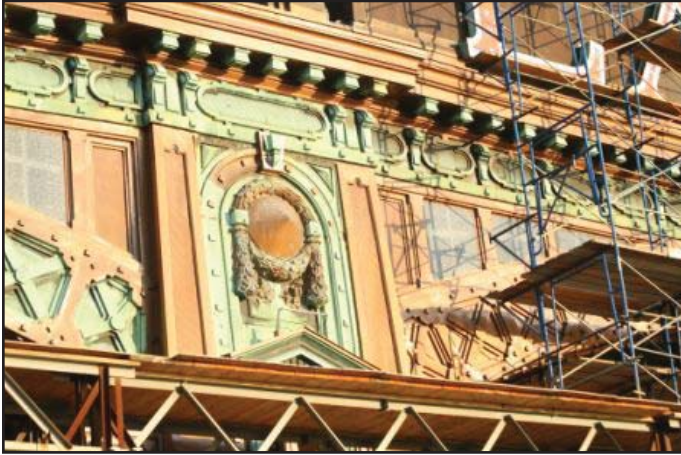
Schtiller & Plevy worked to restore the beauty of decorative architectural elements, which are part of the ferry terminal's unique look.
